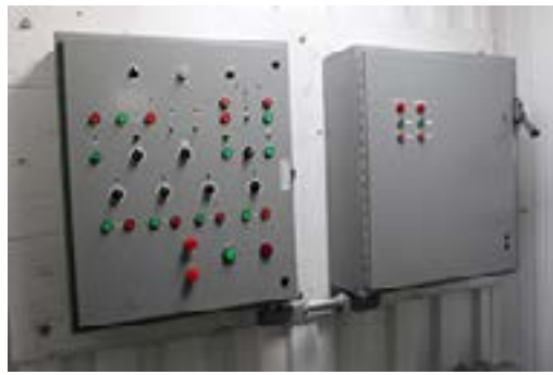
CONTROL SYSTEM ver 1.1
